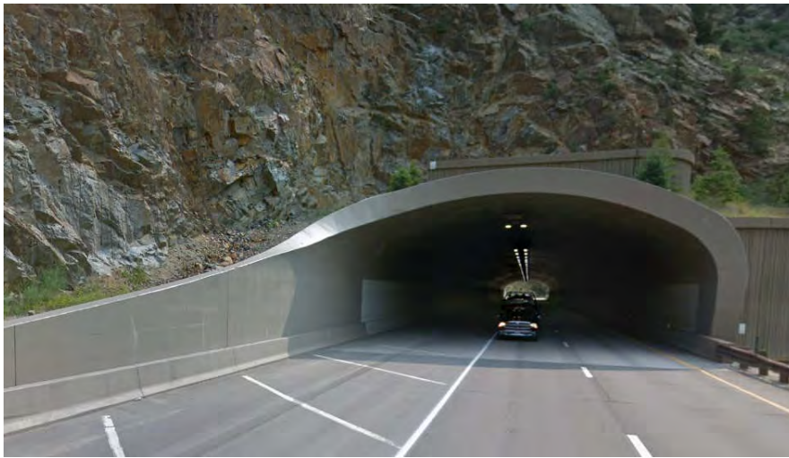
Figure 15.4 - Canopy Structure Used for the Veterans Memorial Tunnels Project for Rockfall Protection
