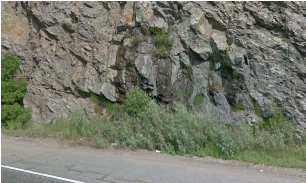
Figure 9. Seepage noted in I-70 rock cut at approximate mile marker 244.2 (Google Earth).
