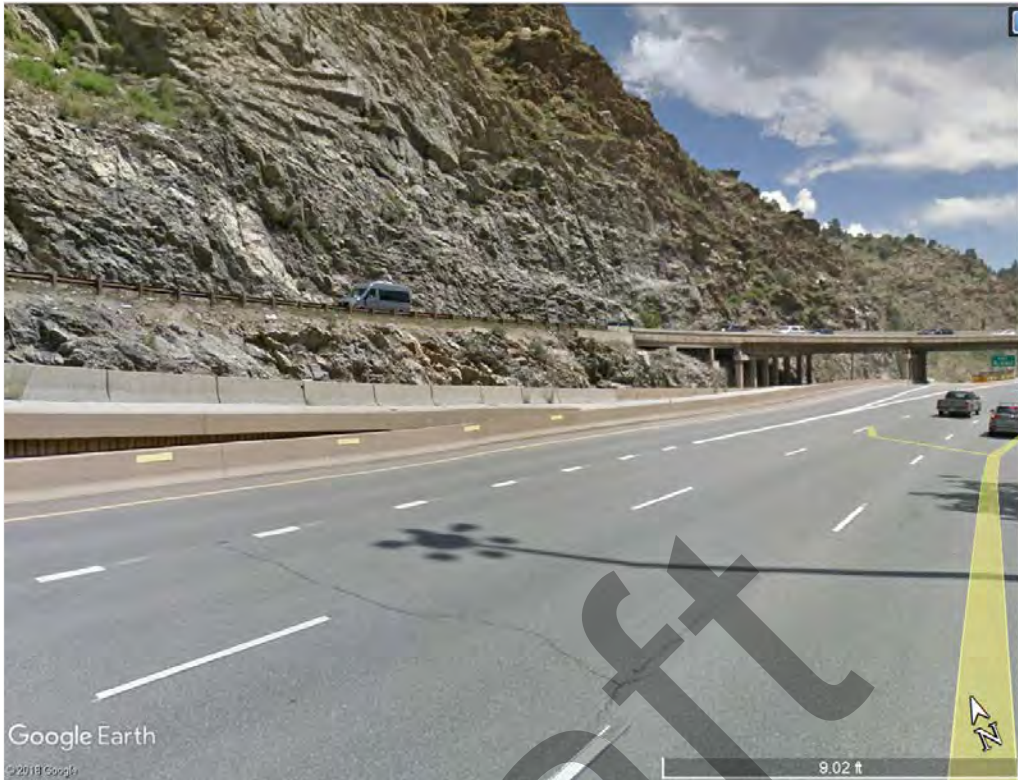
Exhibit 4-1: Bedrock visible from existing I-70 EB bridge over Clear Creek at base of Floyd Hill (image courtesy of Google Earth Pro Street View).
